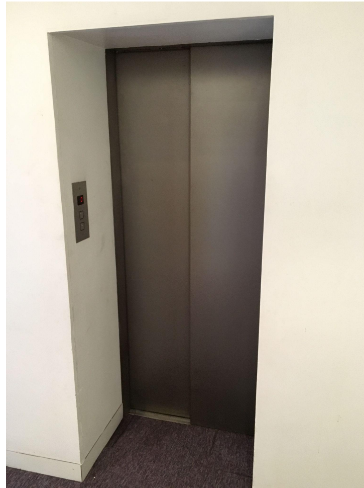
Interior (Basement) Access to lift from basement corridor
